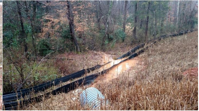
Item #2 – Outlet #2 – fix silt fence or remove it. Photo from 2/12/19.
