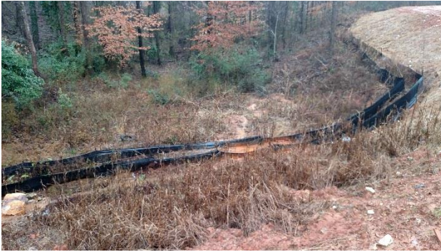
Item #1 – Outlet #1 – fix silt fence or remove. Photo from 2/12/19.
